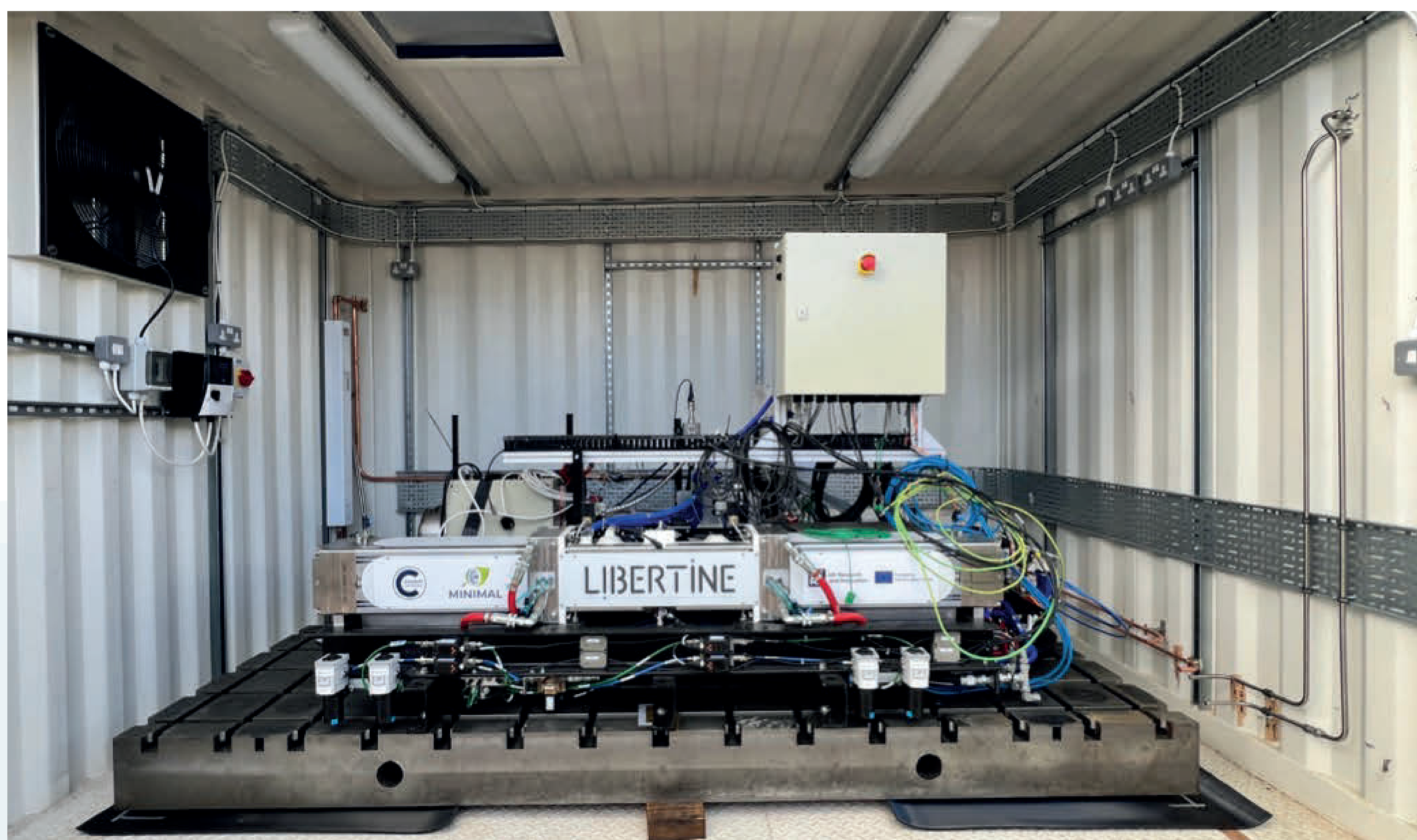
The single cylinder research engine installed in its containerised test cell
